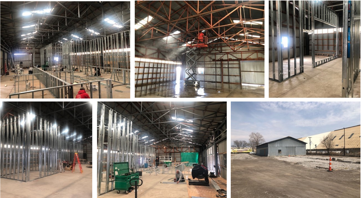
Snapshots of the construction progress at the Eagle Park property as of the end of March.
